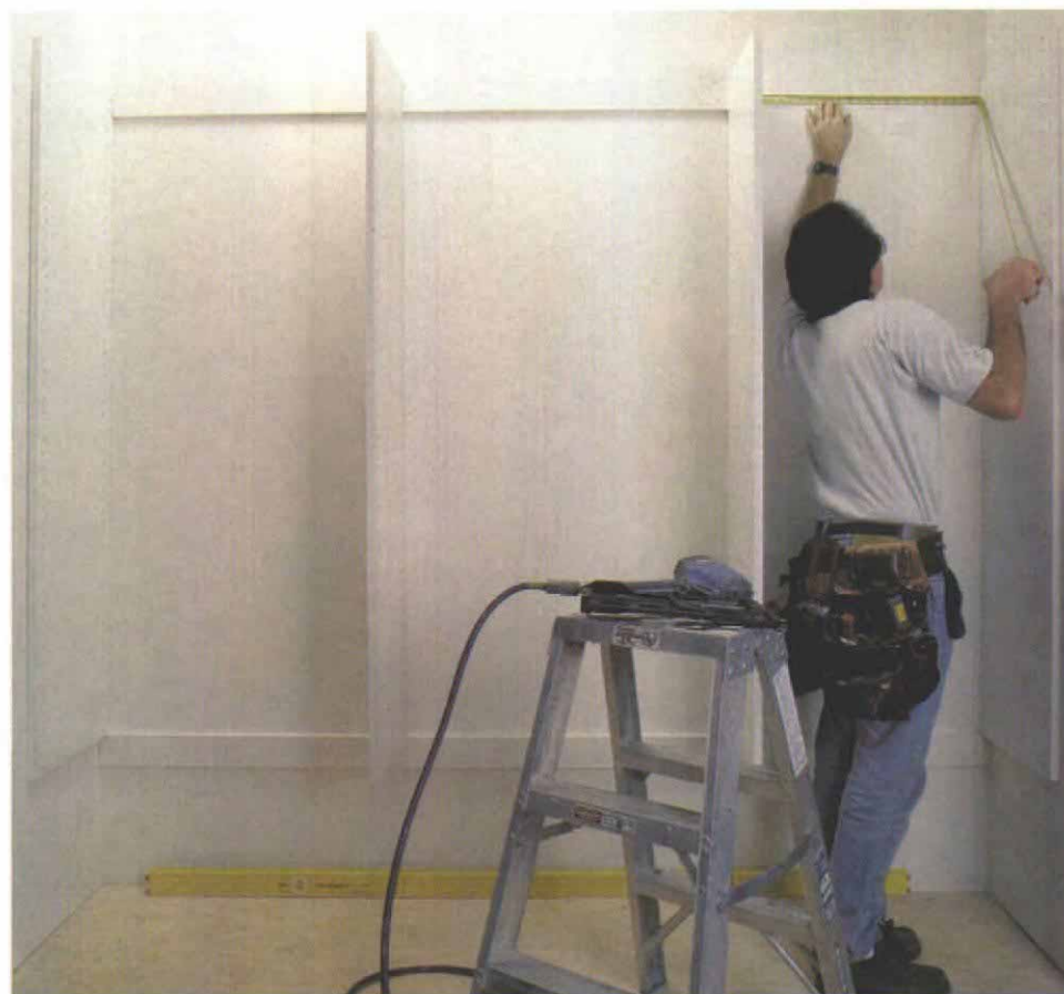
The only measurement in the closet. Other than the initial measurement for the ledger, the only measurement that needs to be taken is for the width of the remaining space. All other measurements are predetermined.
